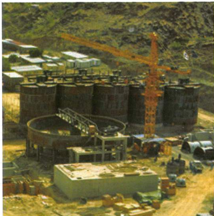
Fig 7 - Pre-Leach Thickener & Leach Tanks
